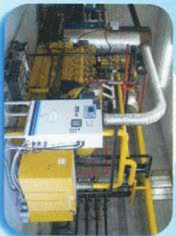
Manure Methane Digester
